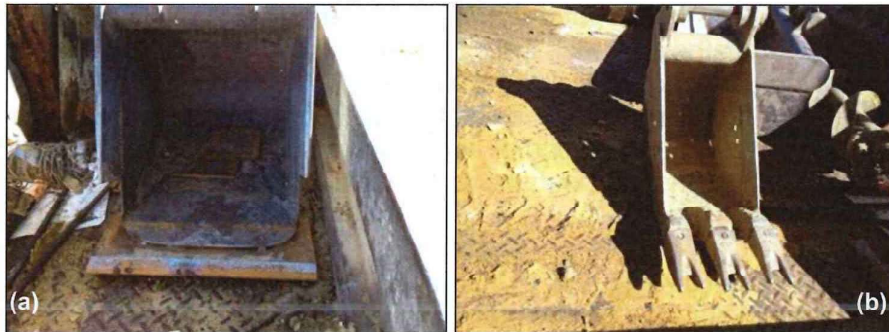
Figure 8. Where mechanical excavation is used outside the tree protection zone the selection of a toothless bucket (a) and use of a spotter can alleviate the extent of damage to the roots as they are revealed, compared with the toothed bucket (b) type which can significantly tear and damage roots.
