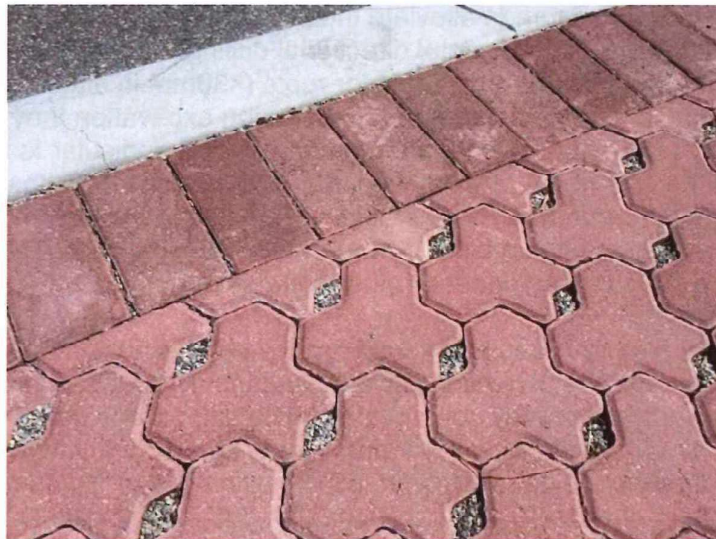
Figure 9. Where hard surfacing is proposed adjacent/ within the TPZ of mature existing trees the use of permeable paving provides an option to alleviate the negative impacts of reduced water infiltration and aeration to the absorbing roots (that are responsible for the uptake of the water and nutrients, and which require oxygen).
