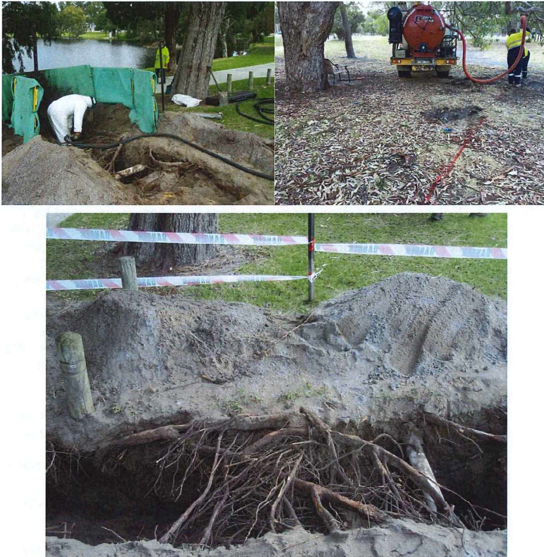
Figure 10. Example of air-spading and soil vacuum to remove soil within the tree protection zone without damaging or severing tree roots, thereby allowing a root-sensitive excavation technique for the installation of below-ground services beneath the rootplate.
