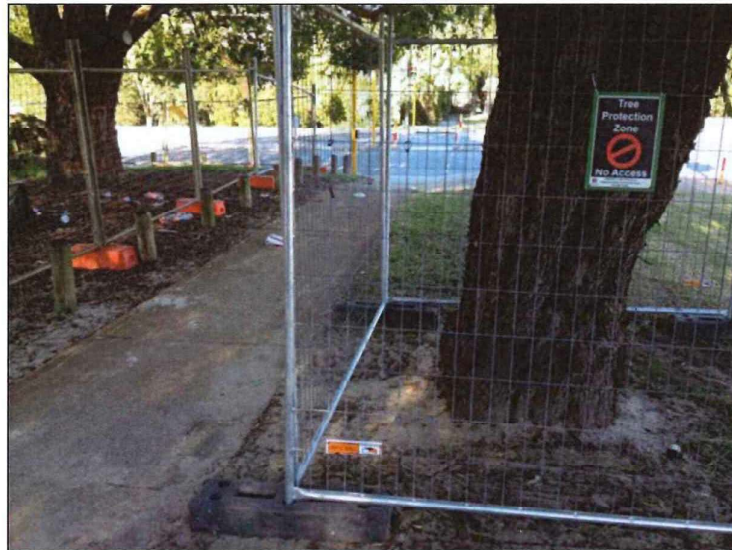
Figure 7. Example of protective fencing comprised of 1.8m high chain-wire mesh panels, which should be erected at the TPZ periphery prior to the commencement of construction activities that have the potential to impact and damage the trunk and lower branches. Due to site constraints typical of a streetscape verge area, the use of four panels (see above) should be considered the minimum tree protection requirement.
